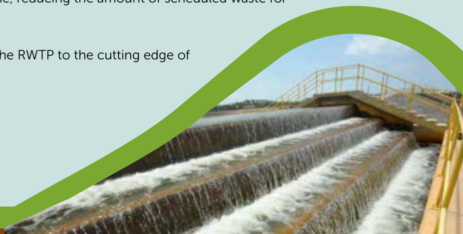
The RWTP efficiently treats 255 MLD of water for PIC through 2 treatment trains for fresh raw water from PAMER and a third train that innovatively recycles storm water
